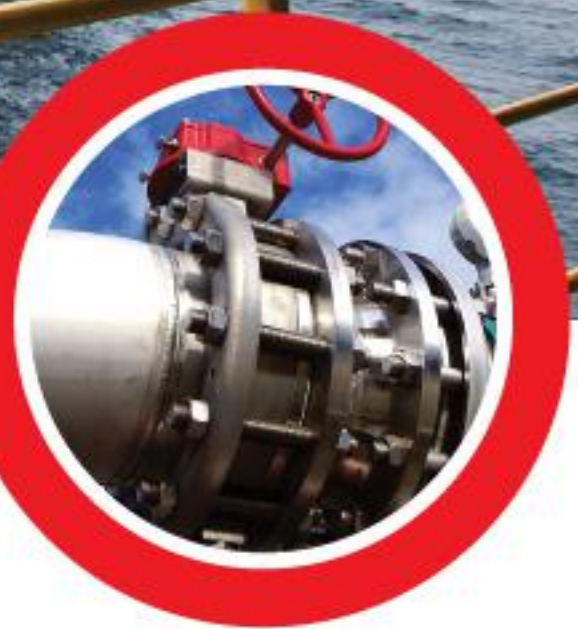
PIPPING & FLUID HANDLING SYSTEMS
